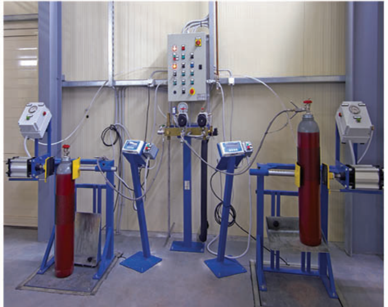
Carbon Dioxide Bottling Department with Four Filling Units
