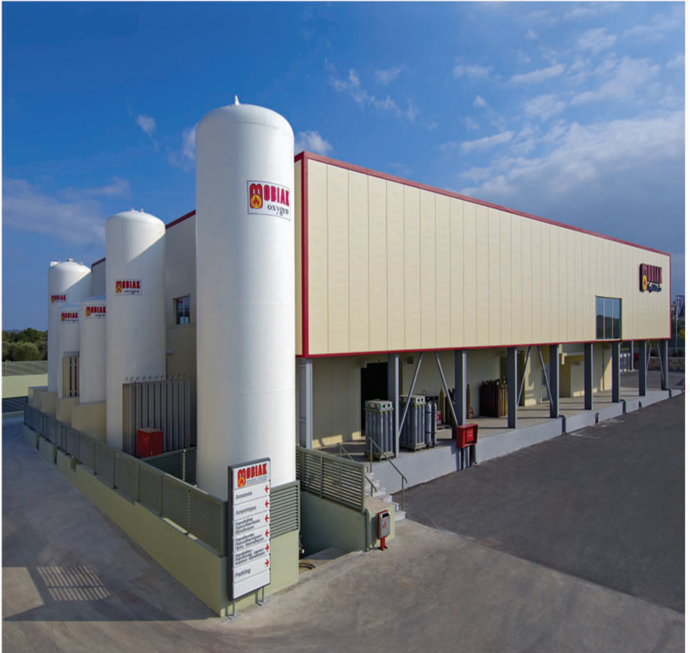
Liquid & Air Sector - Production and Bottling Facilities Cryogenic Tanks are shown in the photo (3 Oxygen, 1 Nitrogen, 1 Argon, 2 Carbon Dioxide)
