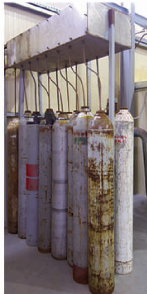
Drying Facility for Cylinders and Extinguishers, following the Hydraulic Test Procedure
